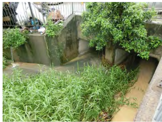
Photo 1 On 13 July 2016, turbid water was observed at WM2B.
