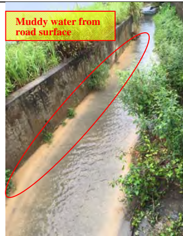
Photo 4 Muddy water was observed flowing from the road surface into the existing channel. The source of muddy water is unknown as it is located outside site boundary.
